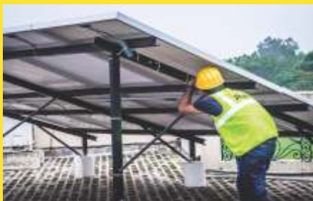
Regular Rooftop installation
